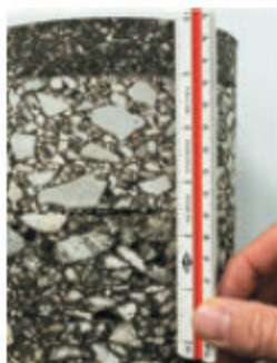
Core showing 1-in. thin asphalt overlay (top)
