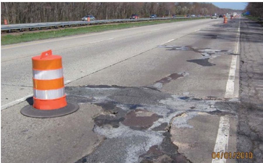
Figure 6.1 Surface Conditions of I-295 JRCP Section from MP 45 to 56.8 in Burlington County (Courtesy of NJDOT)
