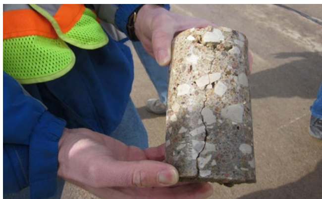
Figure 3.7 Coring for Verifying Through-Slab Cracking (Courtesy of Antigo)
