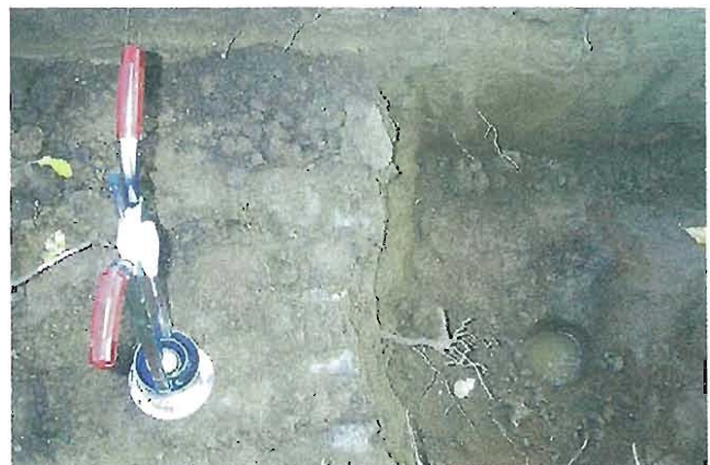
FIGURE 7 The first step in designing any infiltration feature is field investigation of the soils
