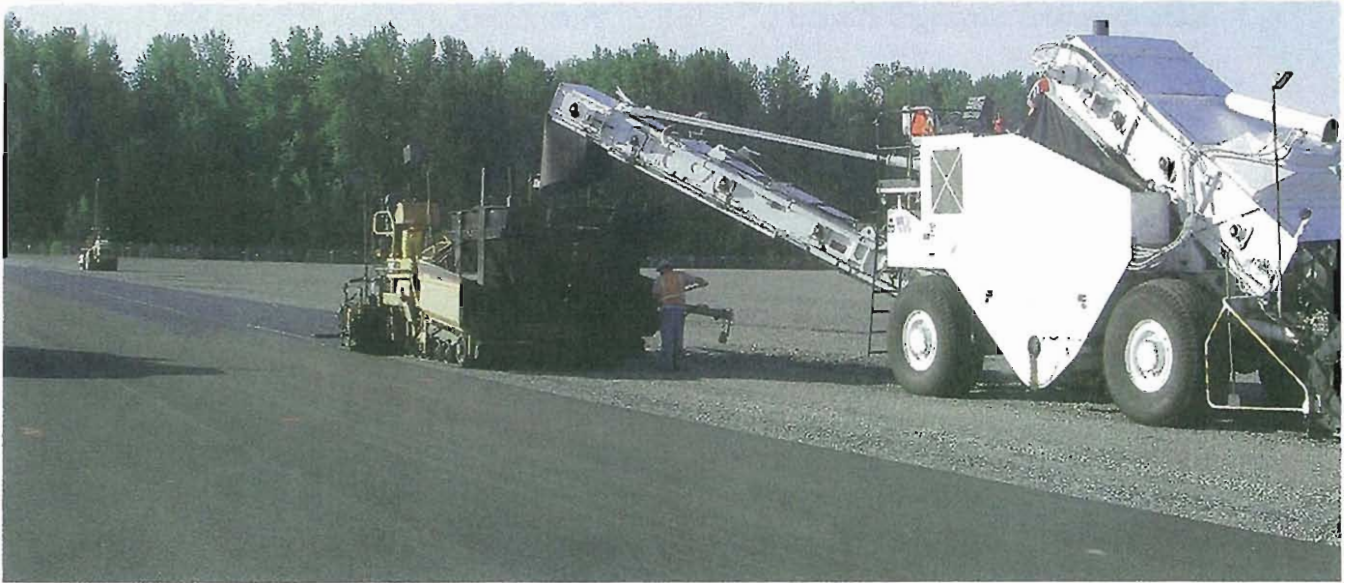
Placing a porous pavement on a large parking lot at the Port of Portland. By using the porous pavement BMP, the Port was able to save time that would have been consumed in the permitting process.
