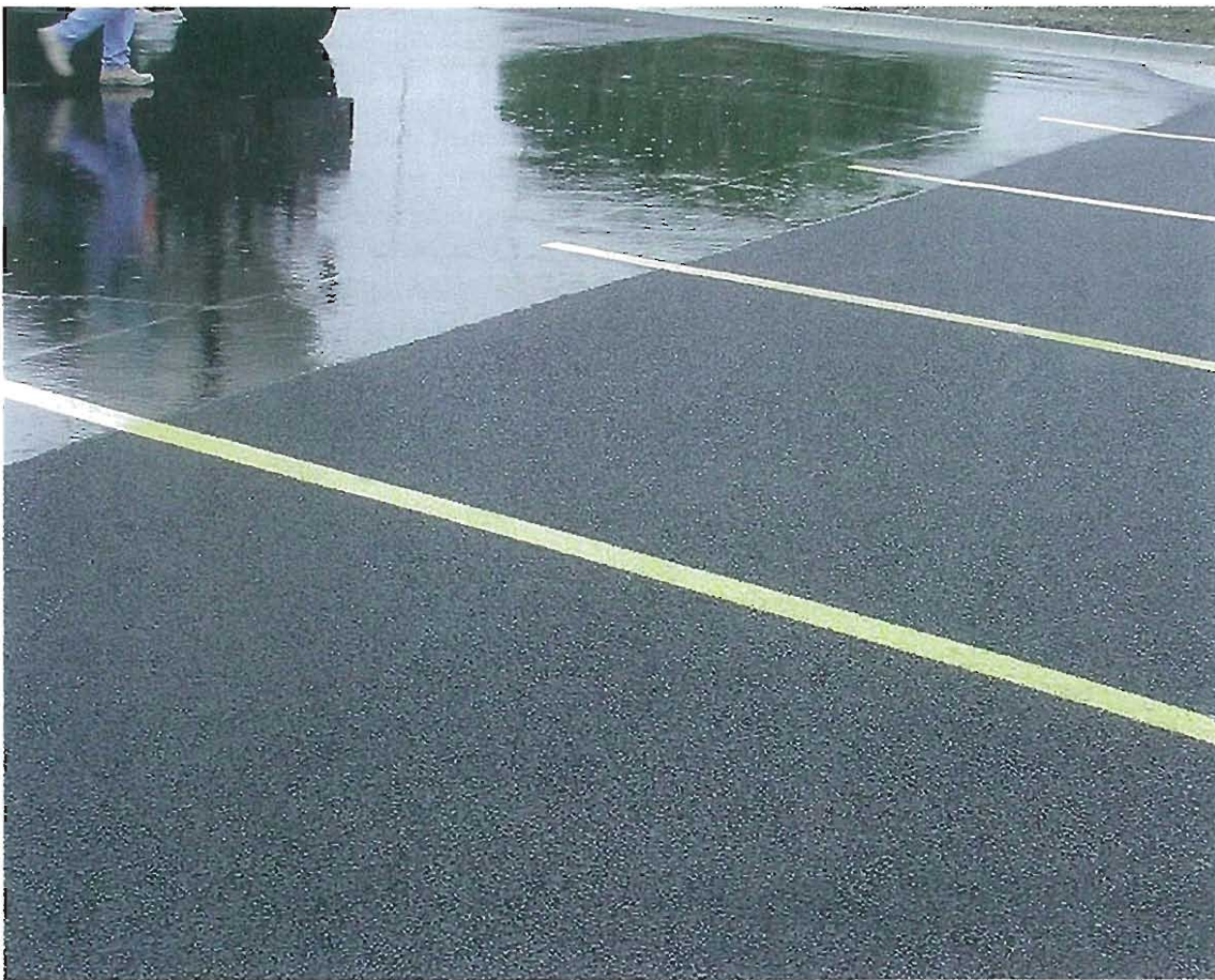
The porous asphalt in the foreground offers a dry surface when a conventional dense-graded asphalt remains wet.
