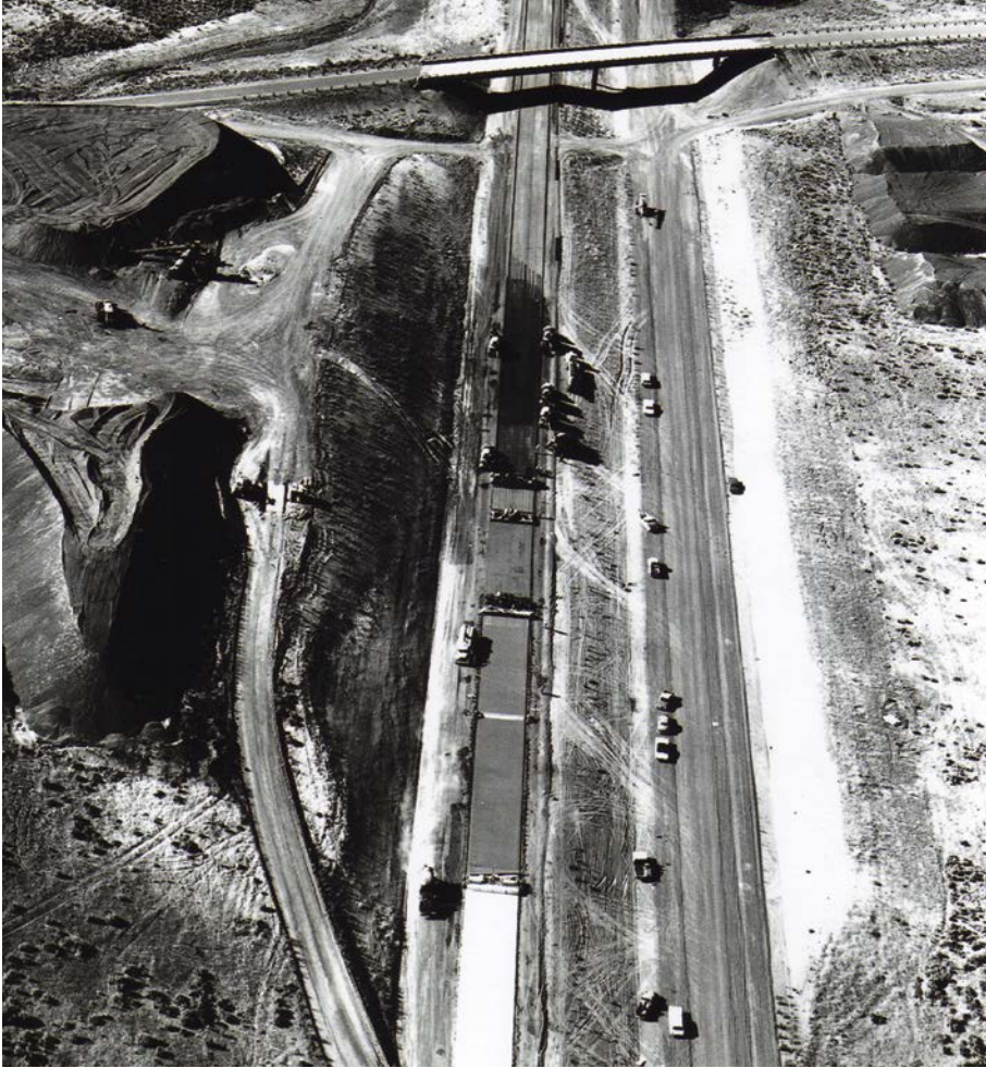
In 1967, construction workers pour pavement on the Huntington Bypass Section of Interstate 84 as work on that section of the interstate system moves steadily toward completion. At this point, Oregon had completed 86% of its Interstate system to present-day standards.
